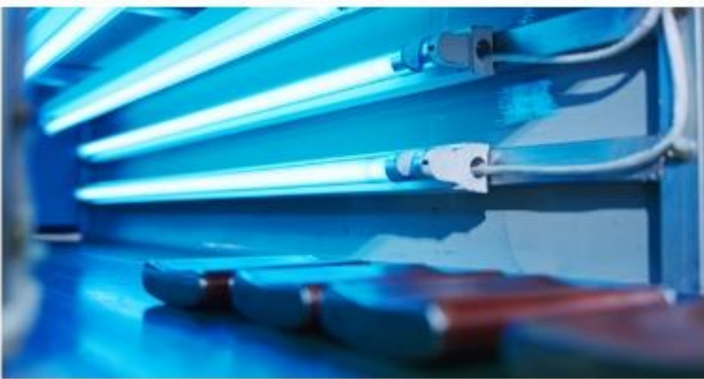
Disinfection by ultraviolet light
